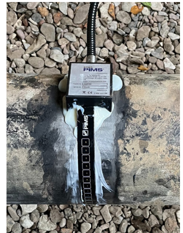
Figure 4: matPIMS™ 1x15 array permanently installed using viscoelastic putty to overcoat sensor strip and head before wrapping/backfill.
