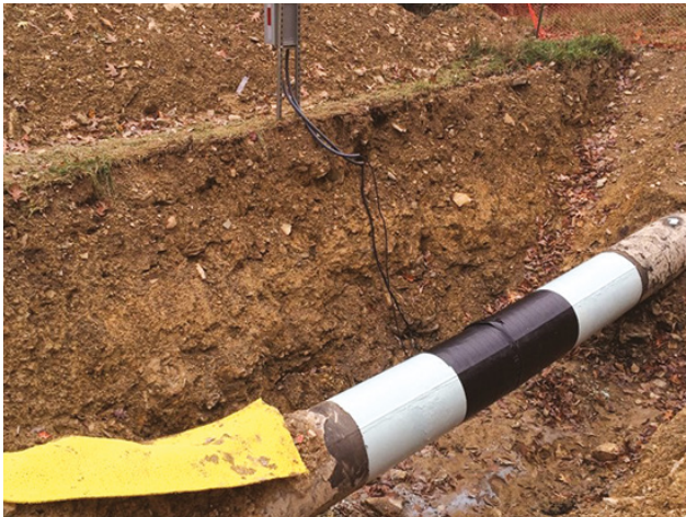
Figure 1: Fully coated and wrapped installation with RS-485 cable mounted in test station for data collection.
